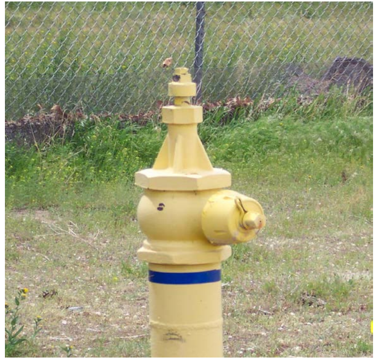
This is a “Jones-Head”. This also is NOT an approved hydrant.
