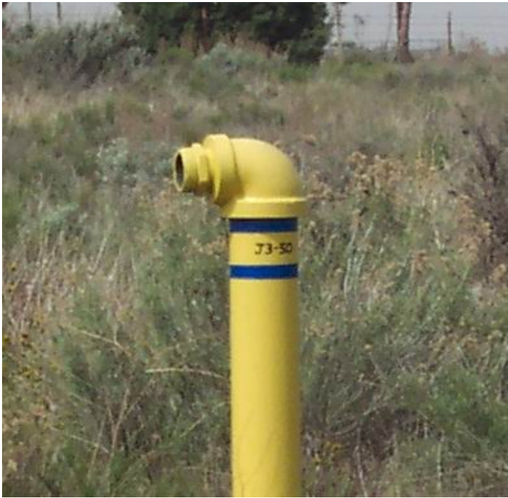
This is a “Blow-Off”. This is NOT an approved hydrant.
