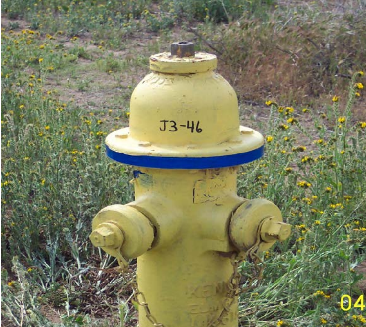
This hydrant is approved for applications requiring Fire Flow of NOT MORE THAN 1000 gpm. Fire Flow letter shall be submitted with application. However, it cannot be installed as a new hydrant
